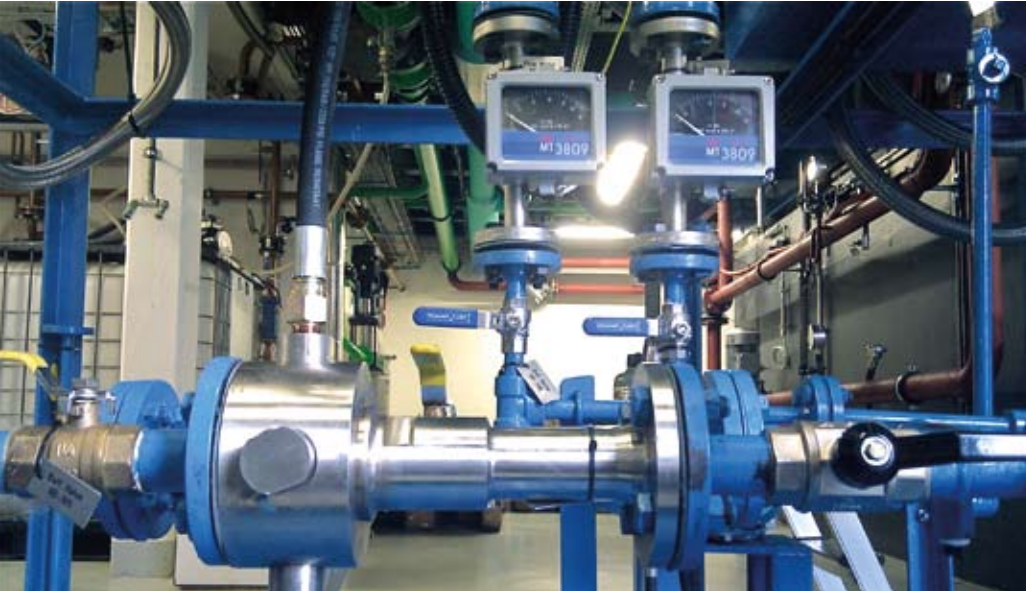
The emulsified fuel technology test facility
