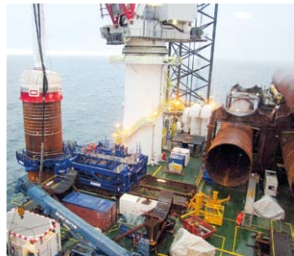
The first monopile being driven into the seabed. The whole operation took 12 hours
